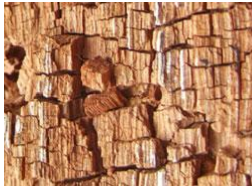
Cubical brown rot ( www.basementsystems.com )
